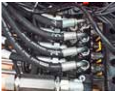
ADVANCED PROPORTIONAL HYDRAULIC SYSTEM
