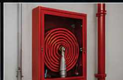
FIRE HYDRANT & WET RISER SYSTEMS
