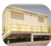
EPIC PROJECT OF 22KV PACKAGE SUBSTATIONS
