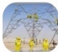
EPIC PROJECT OF EHV OVER HEAD LINES UPTO 400KV
