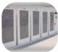
PILOT PROJECT-BATTERY ENERGY STORAGE SYSTEM - TESLA POWERPACK (40MW)
